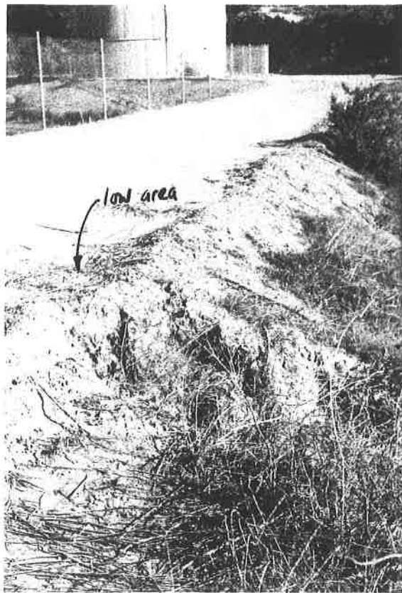
View shows area of low spot in crest and erosion gully on the downstream slope.
